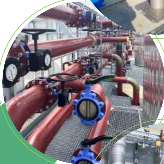
DATA CENTER France
