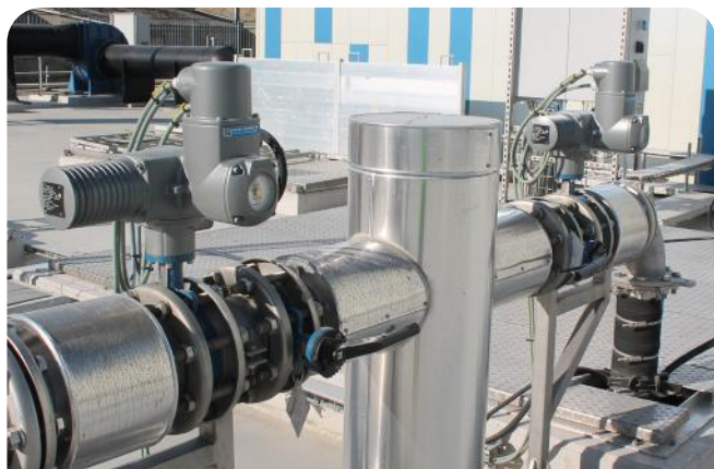
STEP | Eau | BELGIQUE WWTP | Water | BELGIUM
