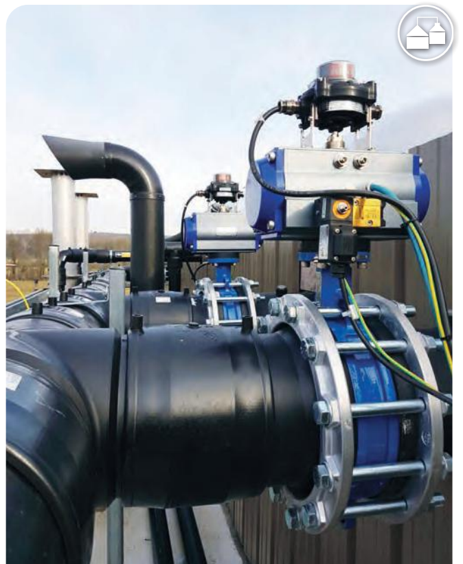
Biogaz | Industrie | FRANCE Biogas - FRANCE
