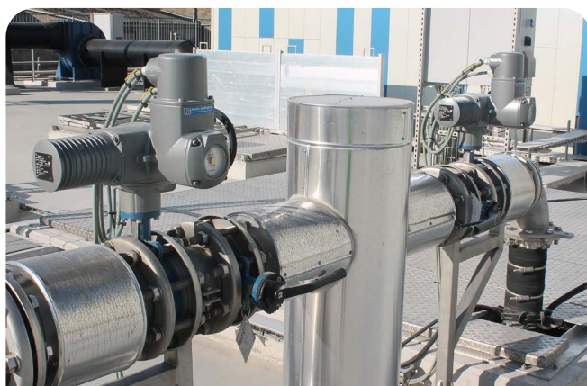
STEP | Eau | BELGIQUE WWTP | Water | BELGIUM
