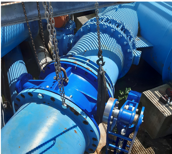
SUEZ - STATION D'EPURATION DE NICE FRANCE
