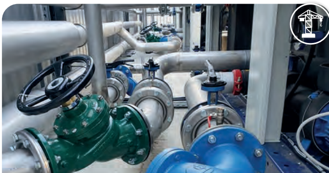
Chaufferie | HVAC | FRANCE Boiler Room - HVAC - FRANCE
