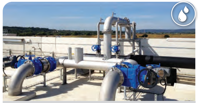
Station d'épuration | Eau | FRANCE Wastewater treatment plant - Water - FRANCE
